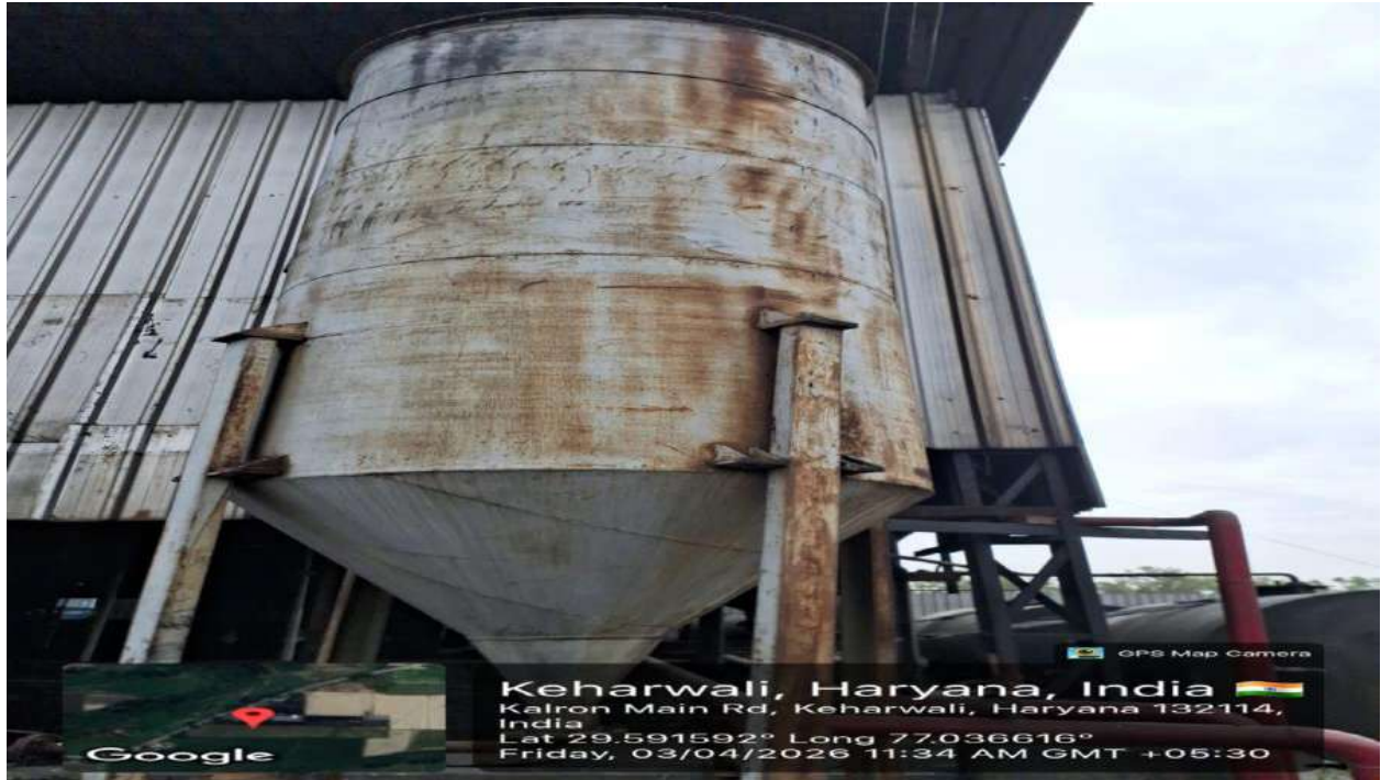
2.4.19 Photograph of separator tank.
