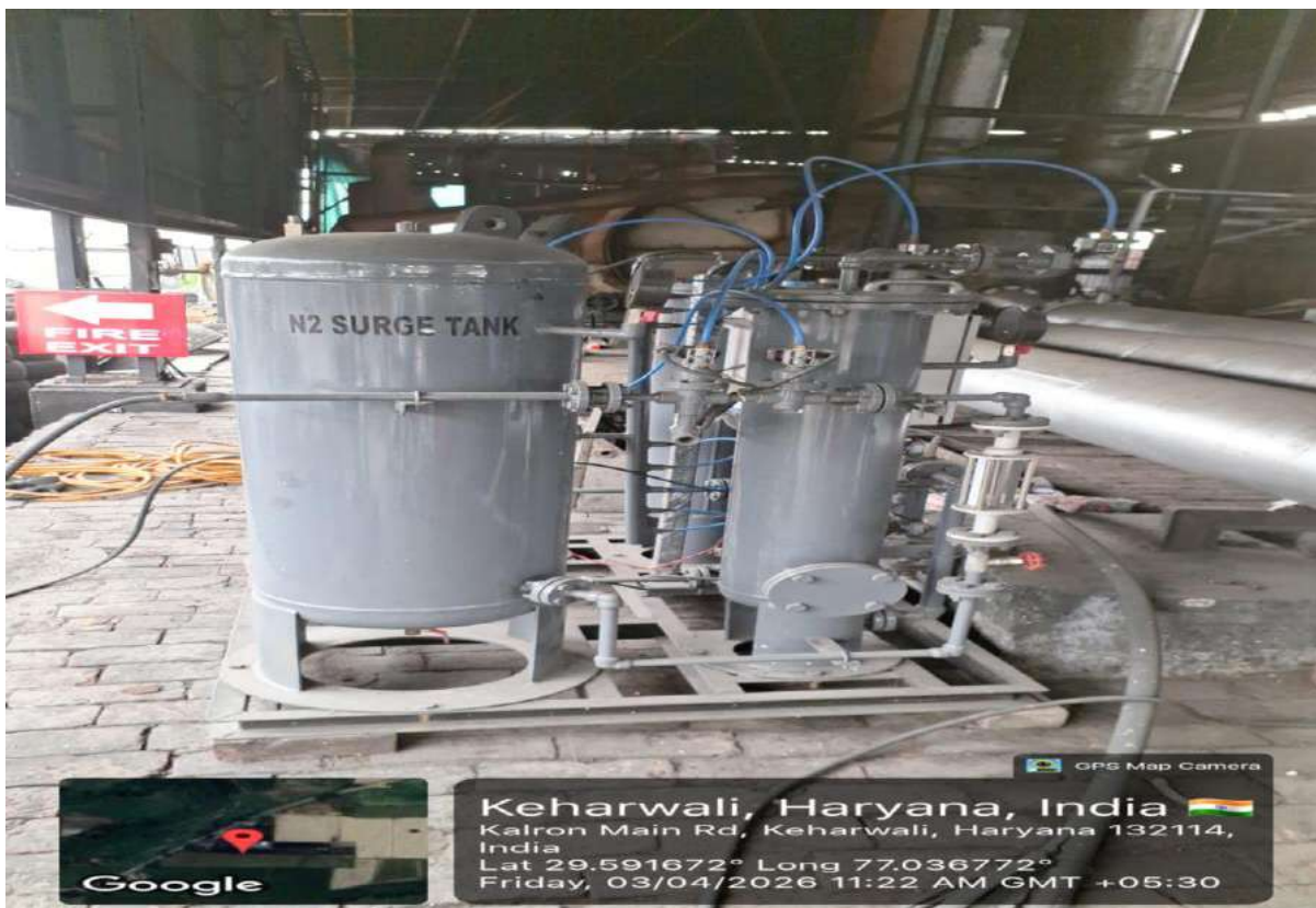
2.4.12 Photograph Nitrogen generator
