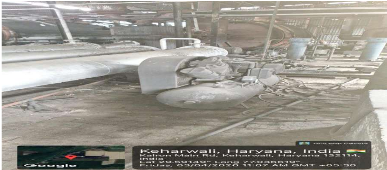
2.4.5 The Photograph of Air compressor
