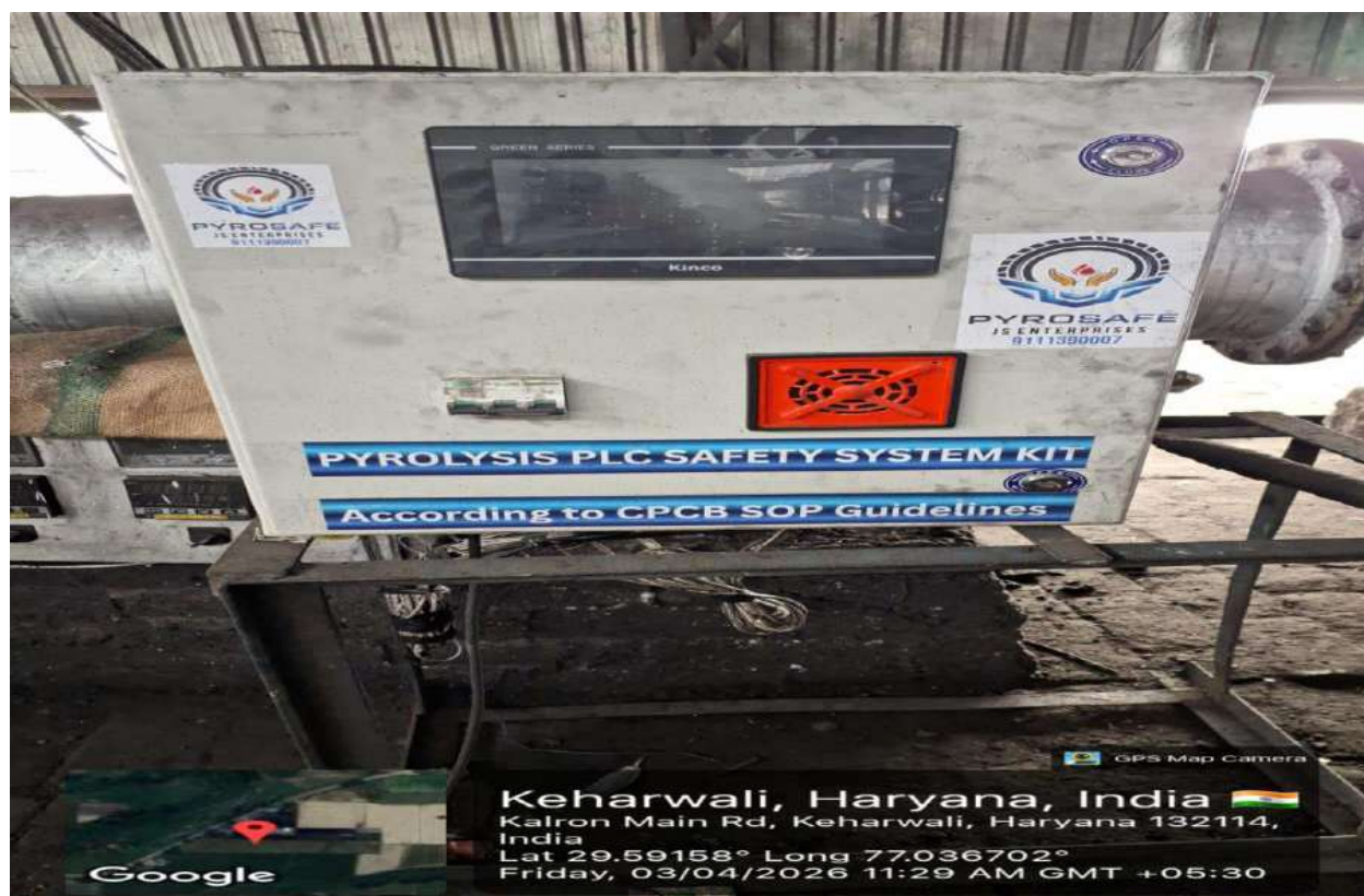
2.4.14 Photograph of Programme Logistic Control (PLC).
