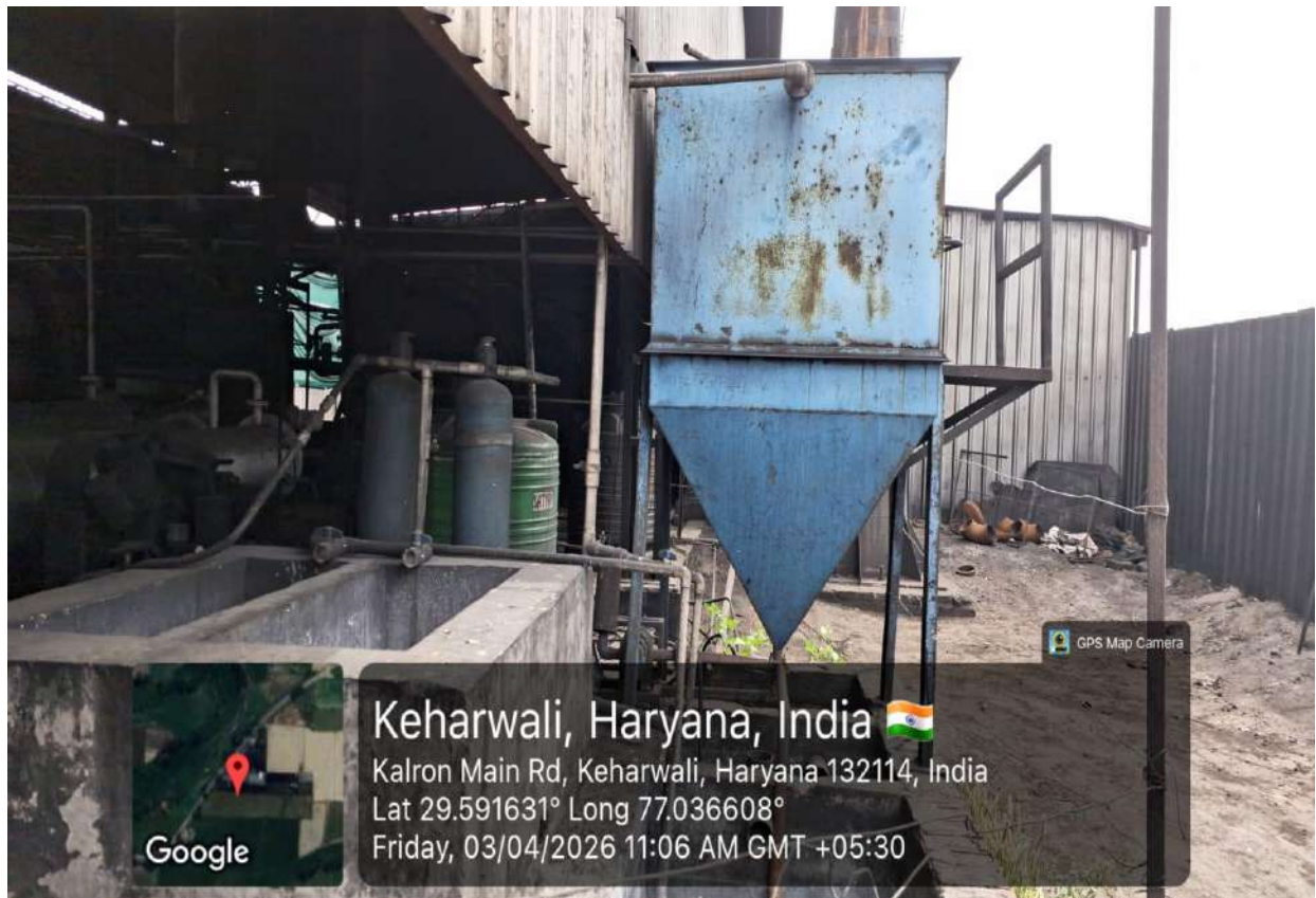
2.4.23 Photograph of ETP.
