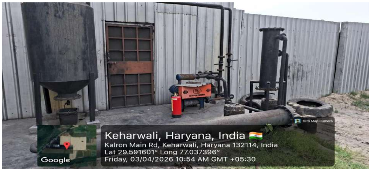
2.4.4 The Photograph of Wet scrubber, Stack and Pyro fuel Storage
